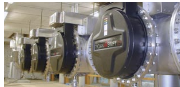
A TrojanUVSwift™ECT system installed at the PWN Water Supply Company in Andijk, the Netherlands.
