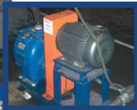
Pump for uptake of wash water behind the screen.
