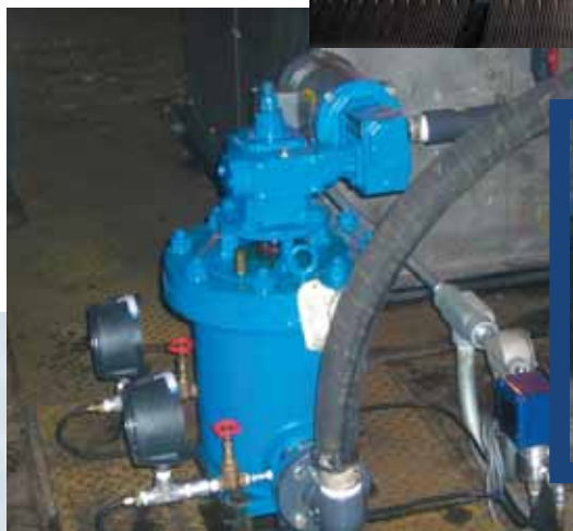
Automatic strainer for wash water
