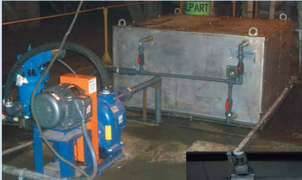
View of screen from grade level. The visible portion of the screen is above the channel. The remainder is below grade level.
