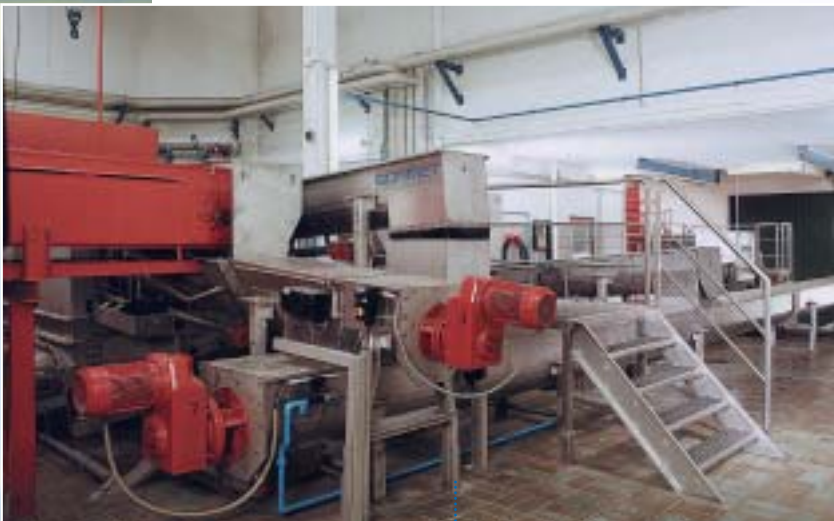
Fine screen with washer/compactor and conveyor system
