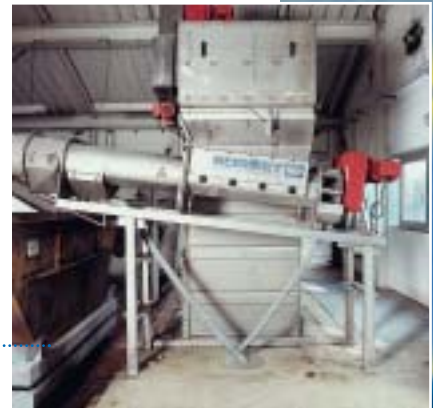
Fine screen with washer / compactor
