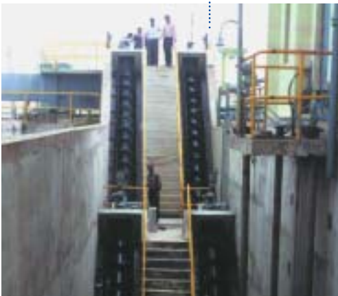
Two stage pumping station
